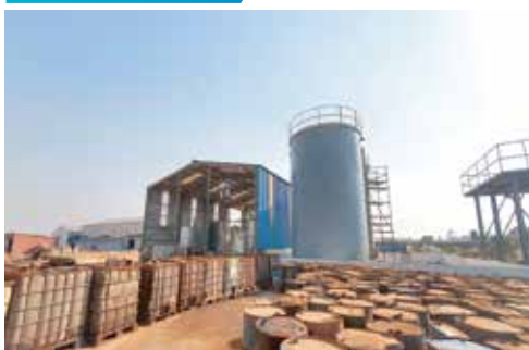
Used Oil Plant
