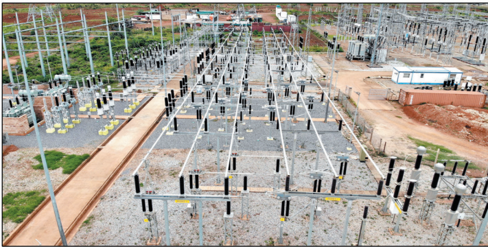
Fungurume - 2x5MVA,120/11 KV Switchyard
