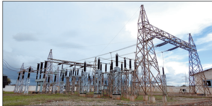
Sotrafer - 1x17.5 MVA, 120/11KV Switchyard
